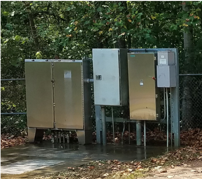
Lift stations at the Flowery Branch facility
